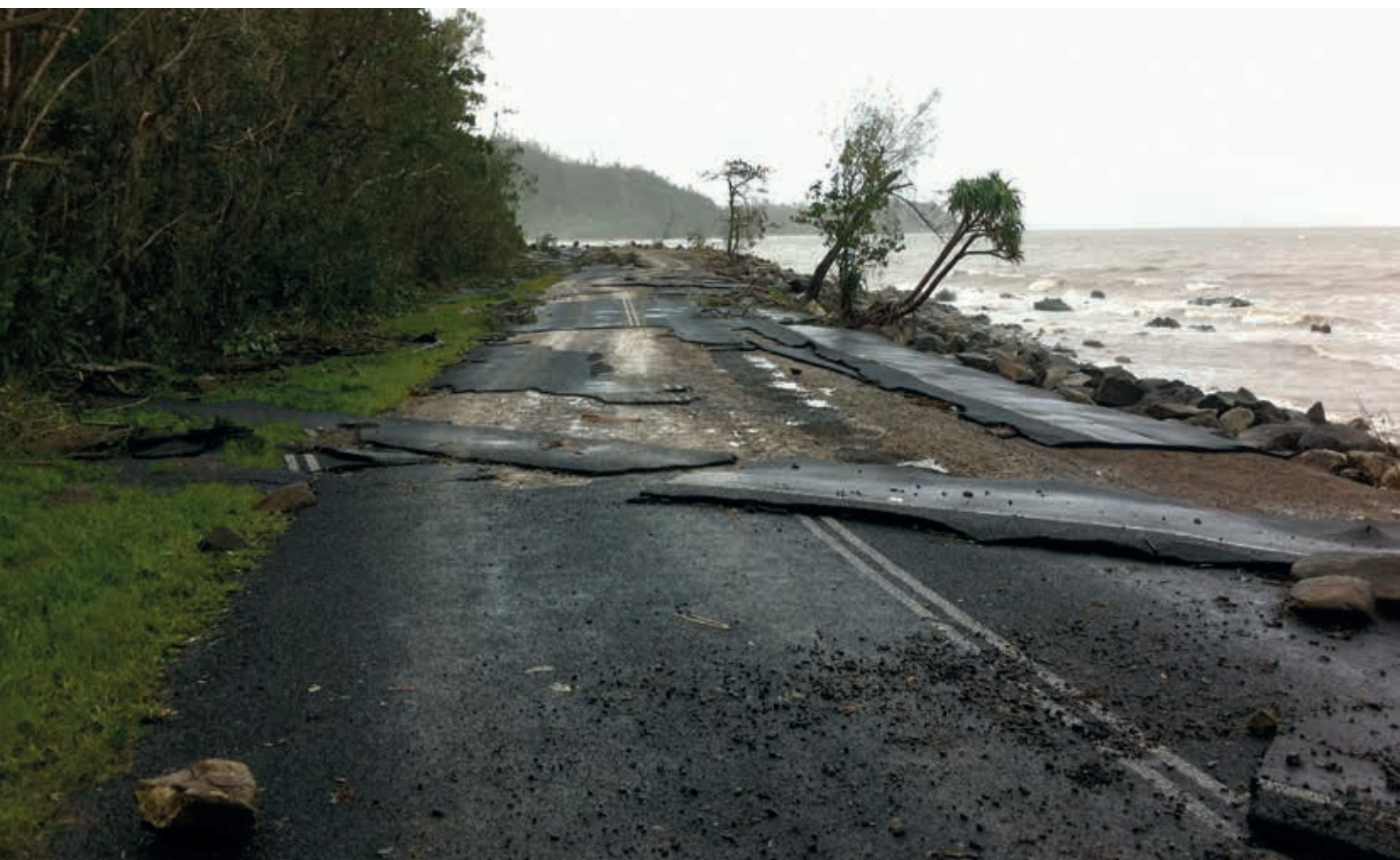
Figure 25: A Queensland road damaged by the impacts of Cyclone Yasi.
