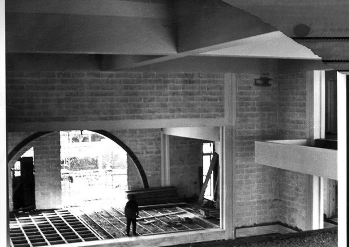
Figure.3- Detail of the construction, Casa da Juventude in Beja. [Raúl Hestnes Ferreira's personal archive]
