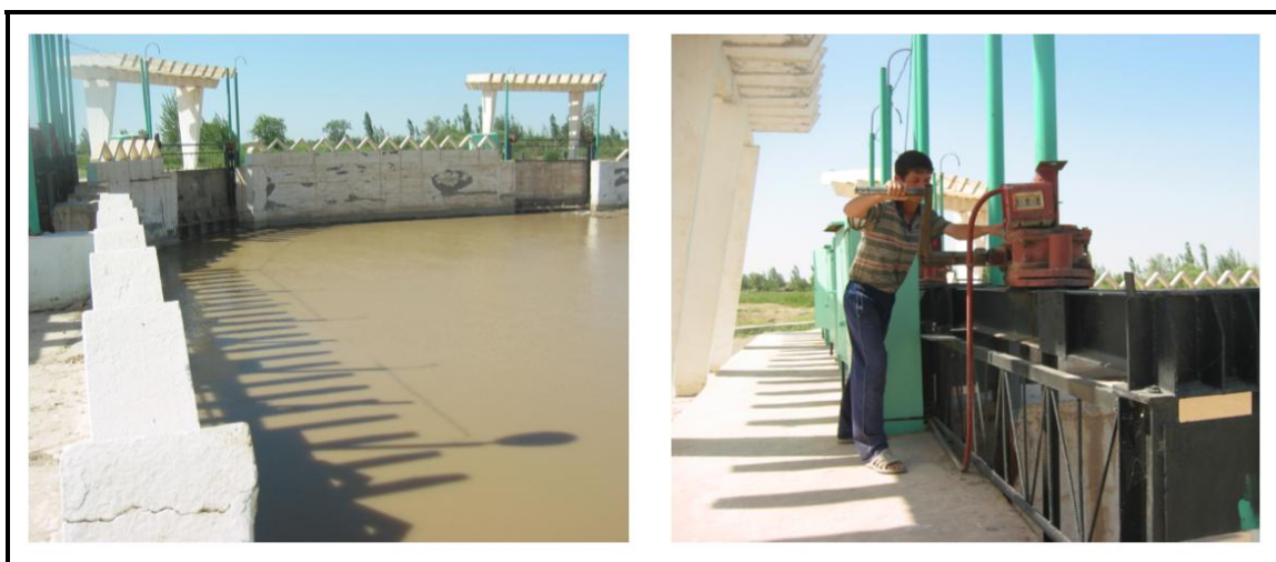
Figure 5.7 – One of the larger water division structures in the R8 system ('Navruz Zaruzenya').
