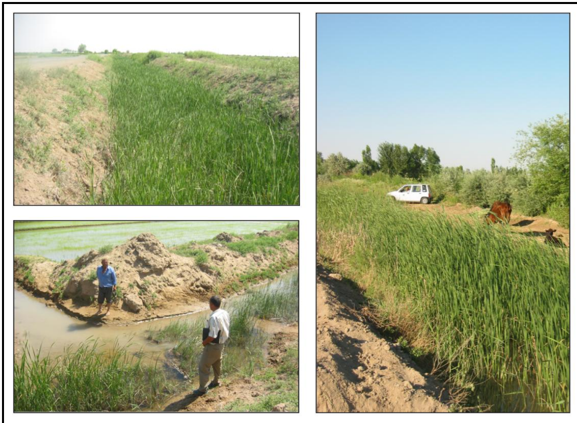
Figure 5.12 – The maintenance state of many drains and collectors is bad
