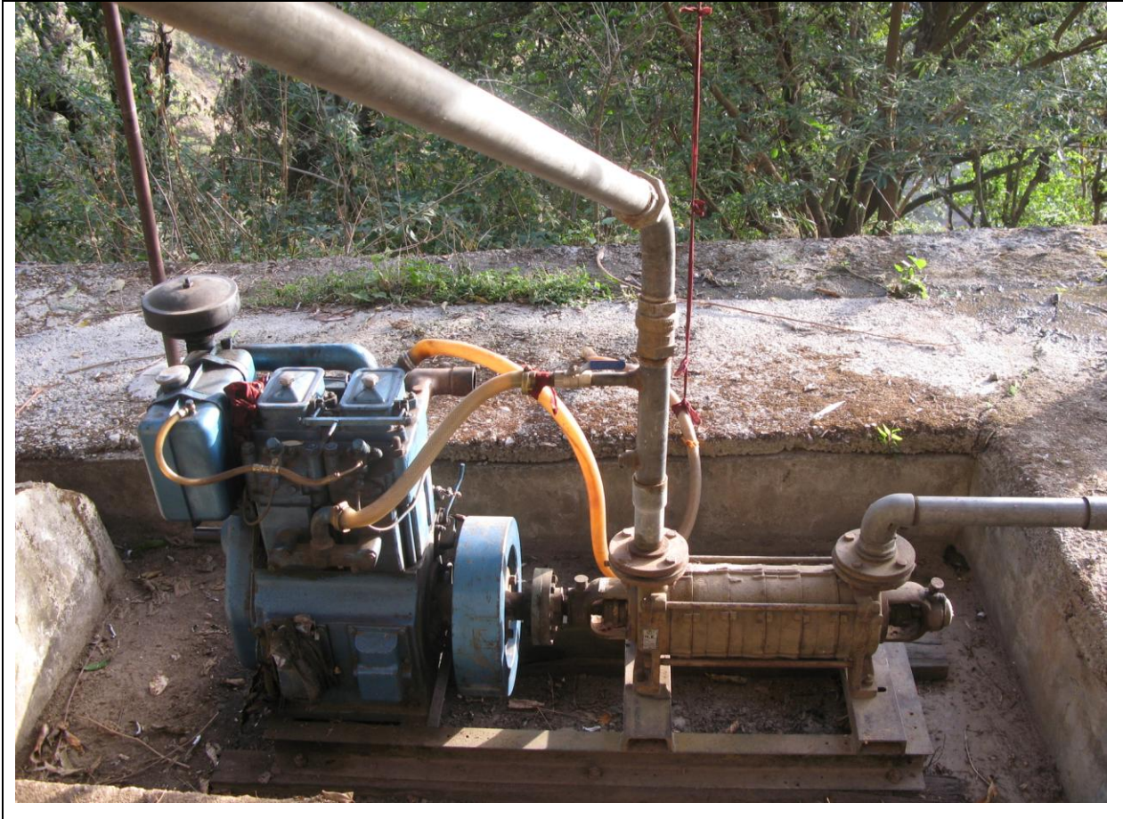
Photograph 2. Diesel Motor Pump in Kimsar Village
