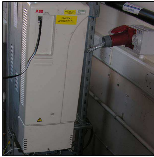
Figure 6.3 Picture of the ABB motor drive system
