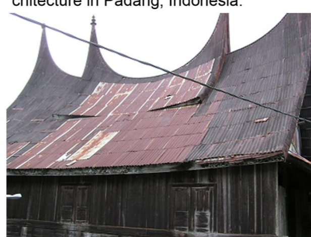
An abundant Minangkabau House in West Sumatra; the house has its original shape of the roof but having non-traditional metal corrugated roofing system.
