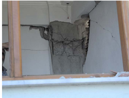
Figure 11. Column with heavy damage.
