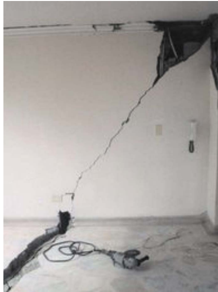
Figure 15. Partitions walls with heavy damage.
