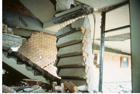
Figure 3. Damage in nonstructural elements, heavy damage in stairs (AIS 2003b).
