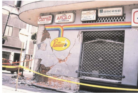
Figure 13. Building of the Coffee-Growing-Region of Colombia damaged by the January 1999 earthquake.
