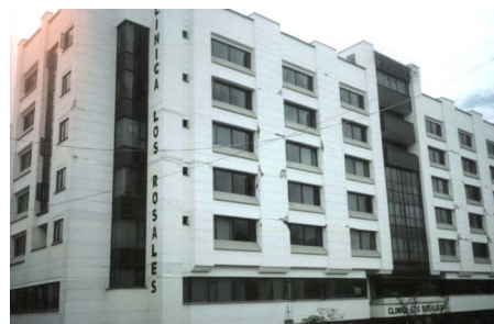
Figure 10. Building of the Coffee-Growing-Region of Colombia damaged by the January 1999 earthquake.
