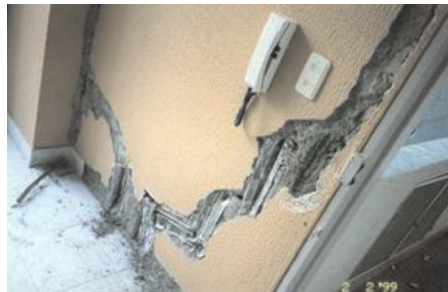
Figure 12. Partitions walls with moderate damage.
