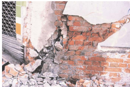
Figure 14. Bearing wall with heavy damage.
