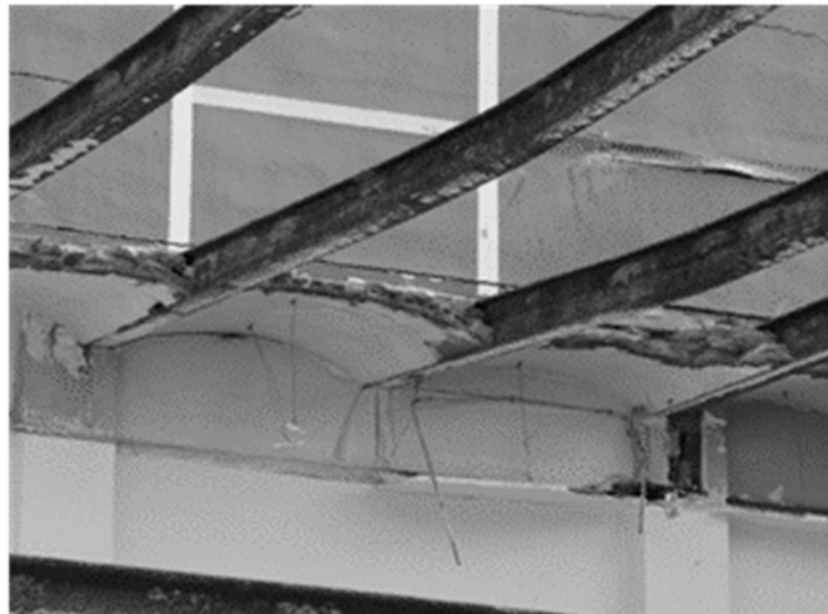
Figure 10. Details of a floor system observed during the demolition of an Eixample building.
