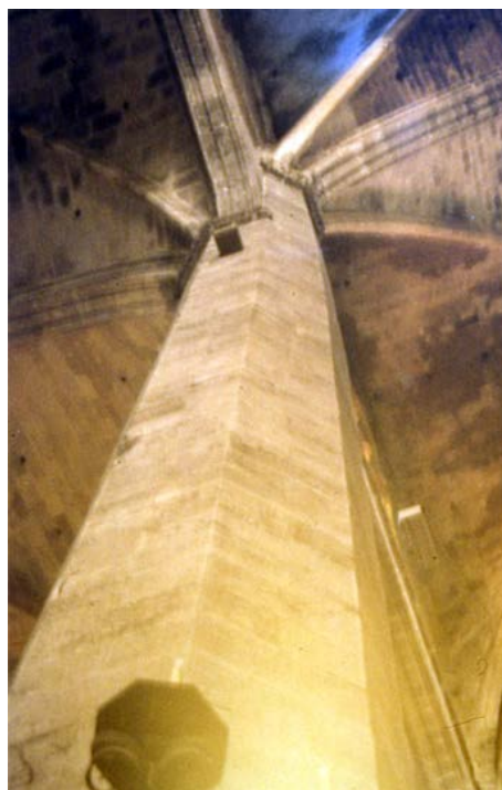
Figure 4 Deformation at the top of a pier.
