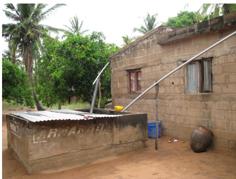
Photo 8 Rainwater structure and tank, Inhambane Province, Mozambique.
