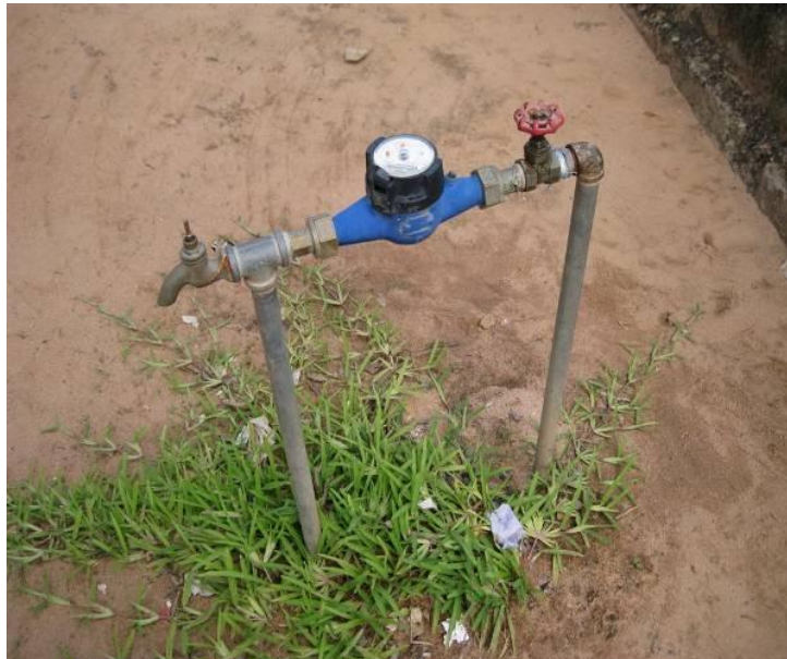
Photo 10 Yard tap with meter, Mozambique.
