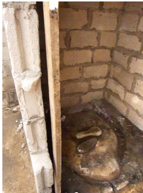
Photograph 1 A dirty and non-used latrine in Mozambique. Photo credit: Peter McIntyre
