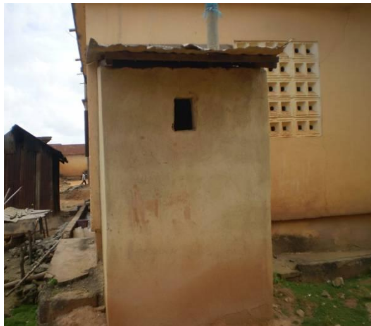
Photo 15 A VIP latrine in Mozambique, defined as having a ventilation shaft, ideally with a fly protector mesh on top
