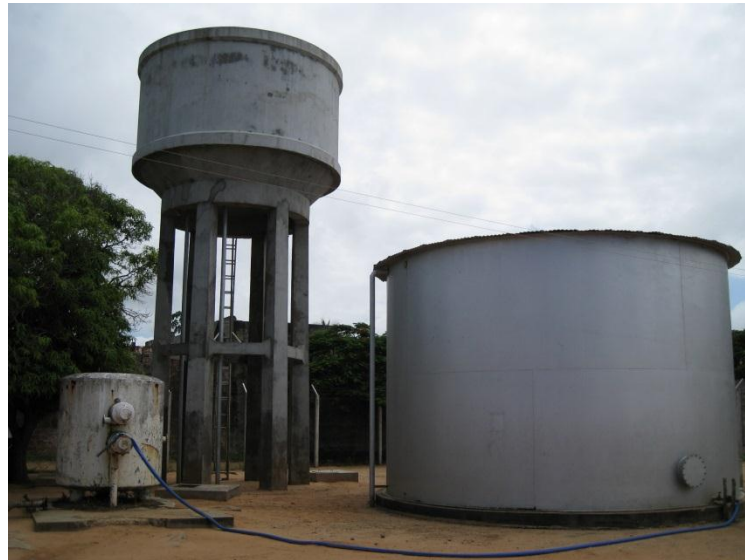
Photo 11 Elevated and ground reservoir feeding small piped systems in Inhambane, Mozambique.
