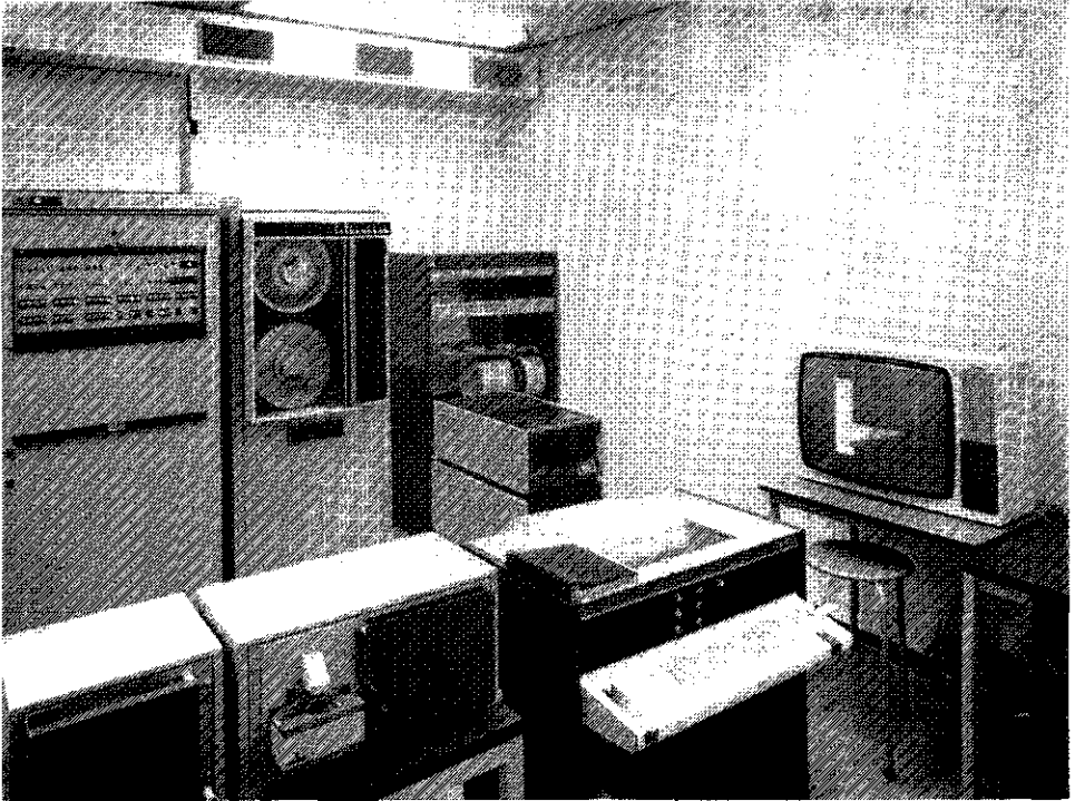
Fig. 4. View of process computer and peripheral units.
