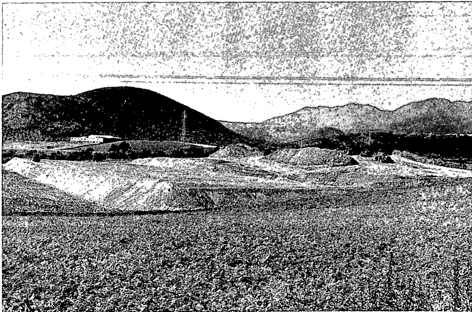
Figure 18.11 Terracing operations in progress for the construction of very large benches. The large step height required to obtain benches large enough for mechanized gravity irrigated agriculture on slopes as steep as 30 percent causes very large volumes of cut and fill (See Figure 9) and requires heavy earthmoving equipment.
