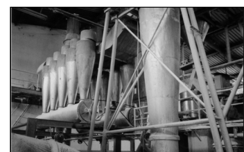
Drying column and hot cyclone
