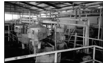
Separator for dewatering process
