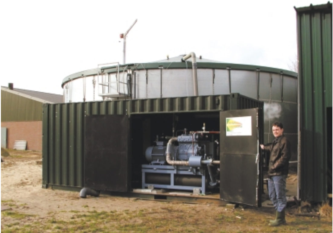
Figure 13. Biogas plant for manure digestion Praktijkcentrum Sterksel, The Netherlands. Photo by courtesy of www.energieprojecten.com .
