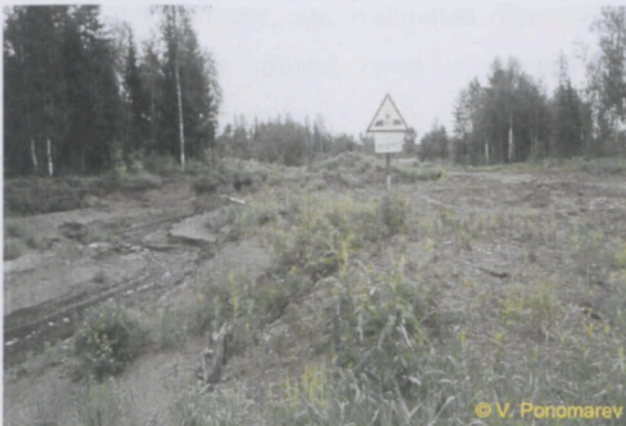
Soil erosion following pipeline construction, Central Vel'yu basin
