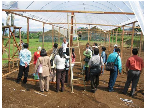
Figure 28. Building the wooden house and explaining its advantages to the course participants, May 2004.
