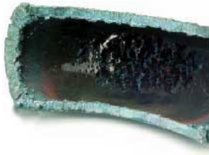
Fig. 16. Erosion and corrosion effects, Source [86]
