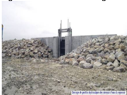
Figure 26.3 Water level management gate
