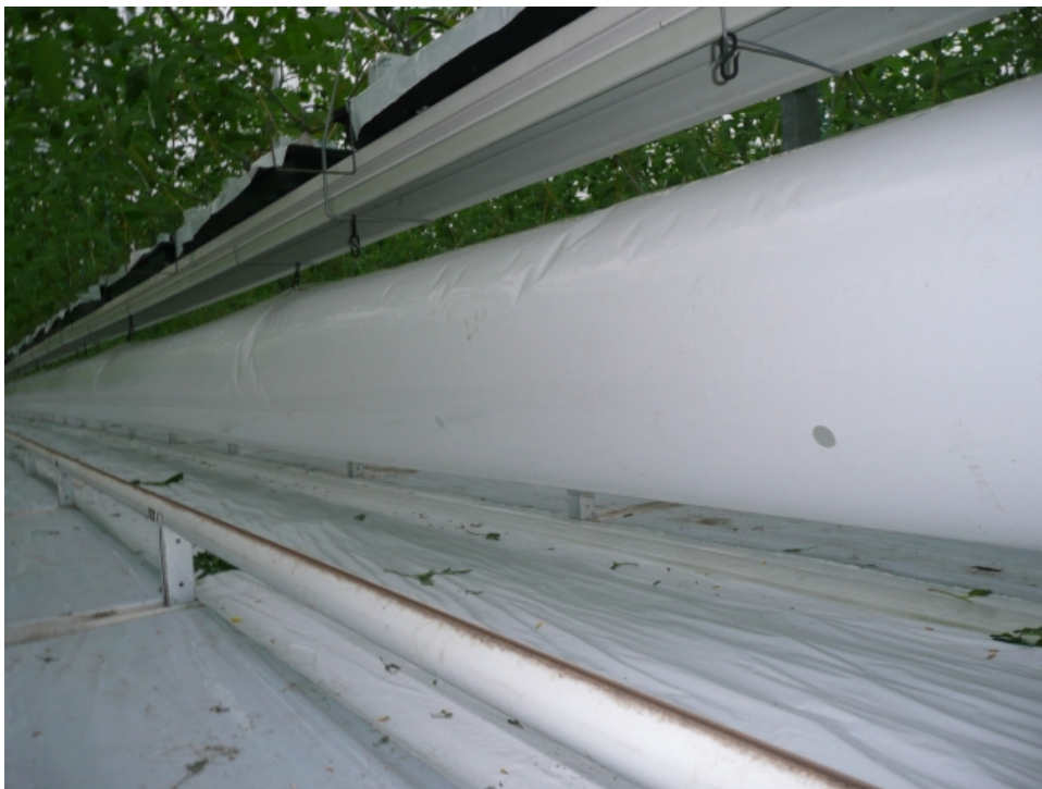
Figure 6.7 Picture of the air duct installed in the greenhouse
