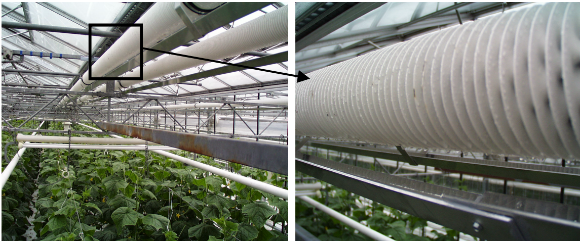
Figure 2.3 Photograph of the greenhouse where finned tubes are placed under the gutter and an enlargement of a finned tube with condensation on the surface.
