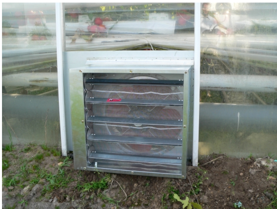
Figure 6.6 Picture of one of the ventilators installed in the side wall of the greenhouse
