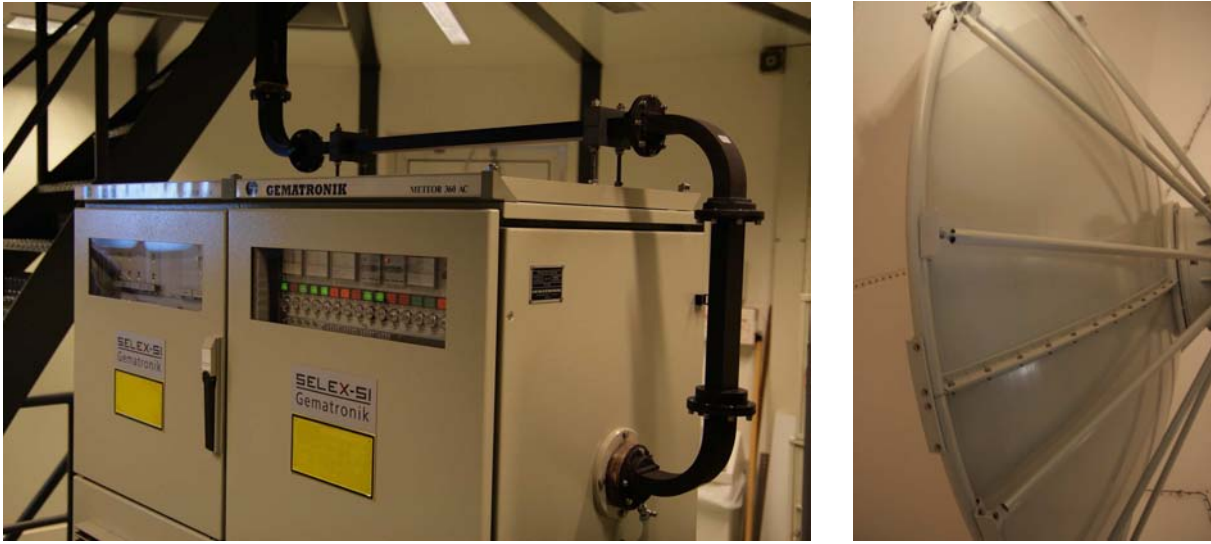
Figure 1.5: Transmitter cabinet, receiver cabinet and waveguide (left), and the circular parabolic reflector of the KNMI weather radar in De Bilt.
