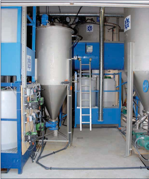
Figure 7 - Anaerobic treatment of black waste(water) in The Netherlands , 32 houses (Meulman, Landustrie BV).
