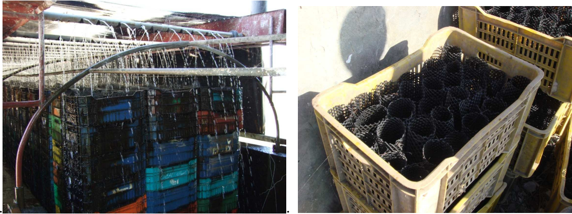
Self-made trickling filter and detail of filter material in recirculation system at the farm of Dr Radwan
