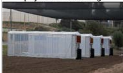
Evaporative cooling F-Clean Covering
