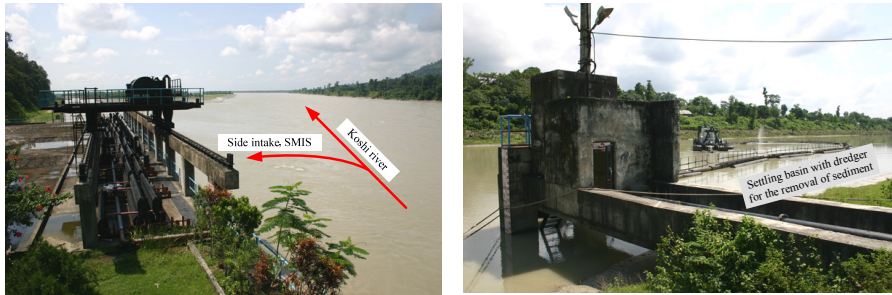
Figure 2.4 Relocated side intake (left) and the settling basin with continuous sediment removal arrangements (right).
