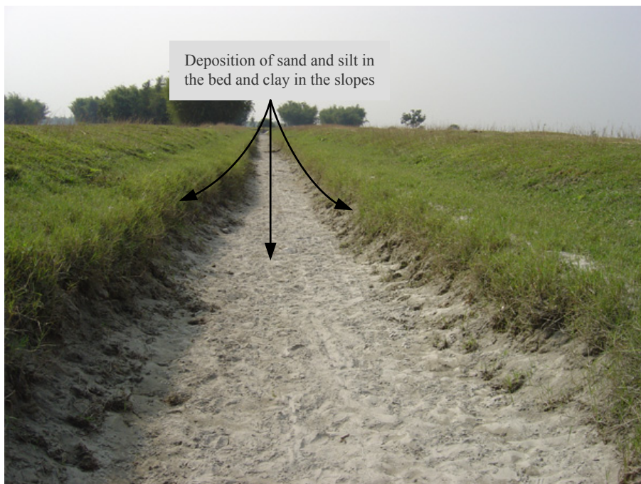
Figure 8.21 Sediment deposition pattern in sub-secondary and tertiary canals.
