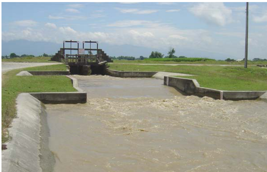
Figure 7.9 Broad crested weir near the intake of Secondary Canal S9 canal for flow measurement.
