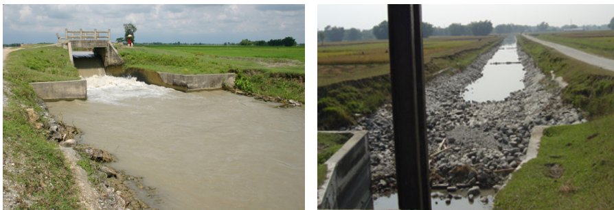
Figure 8.17 Protection work downstream of a water level regulator in Secondary Canal S9.
