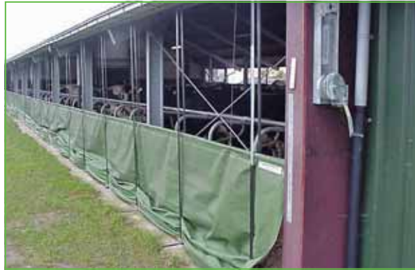
Picture 1. Open side wall combined with a windbreak curtain
