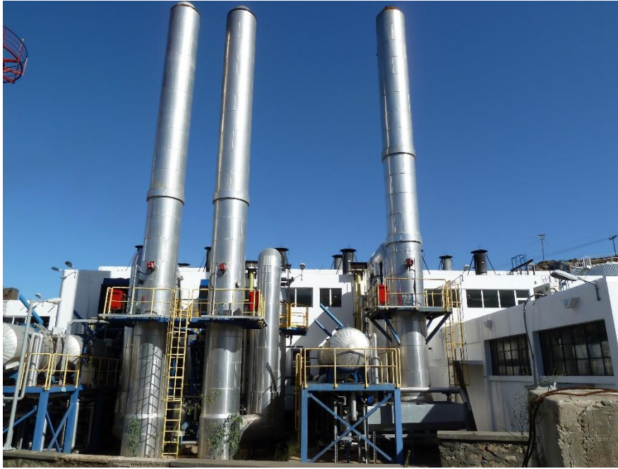
Figure 3-8: Genset stacks and auxiliary equipment
