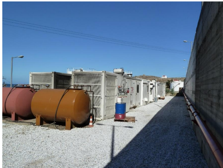
Figure 2-21: Typical mobile Genset and the associated daily fuel tank
