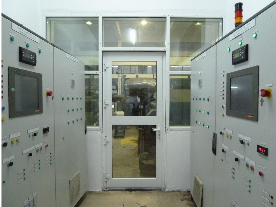
Figure 2-3: Genset Local control room
