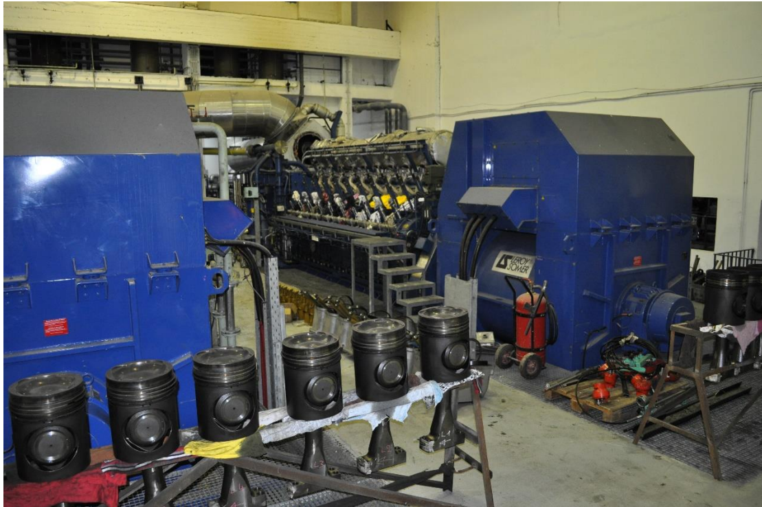
Figure 2-1: Stationary Genset under maintenance
