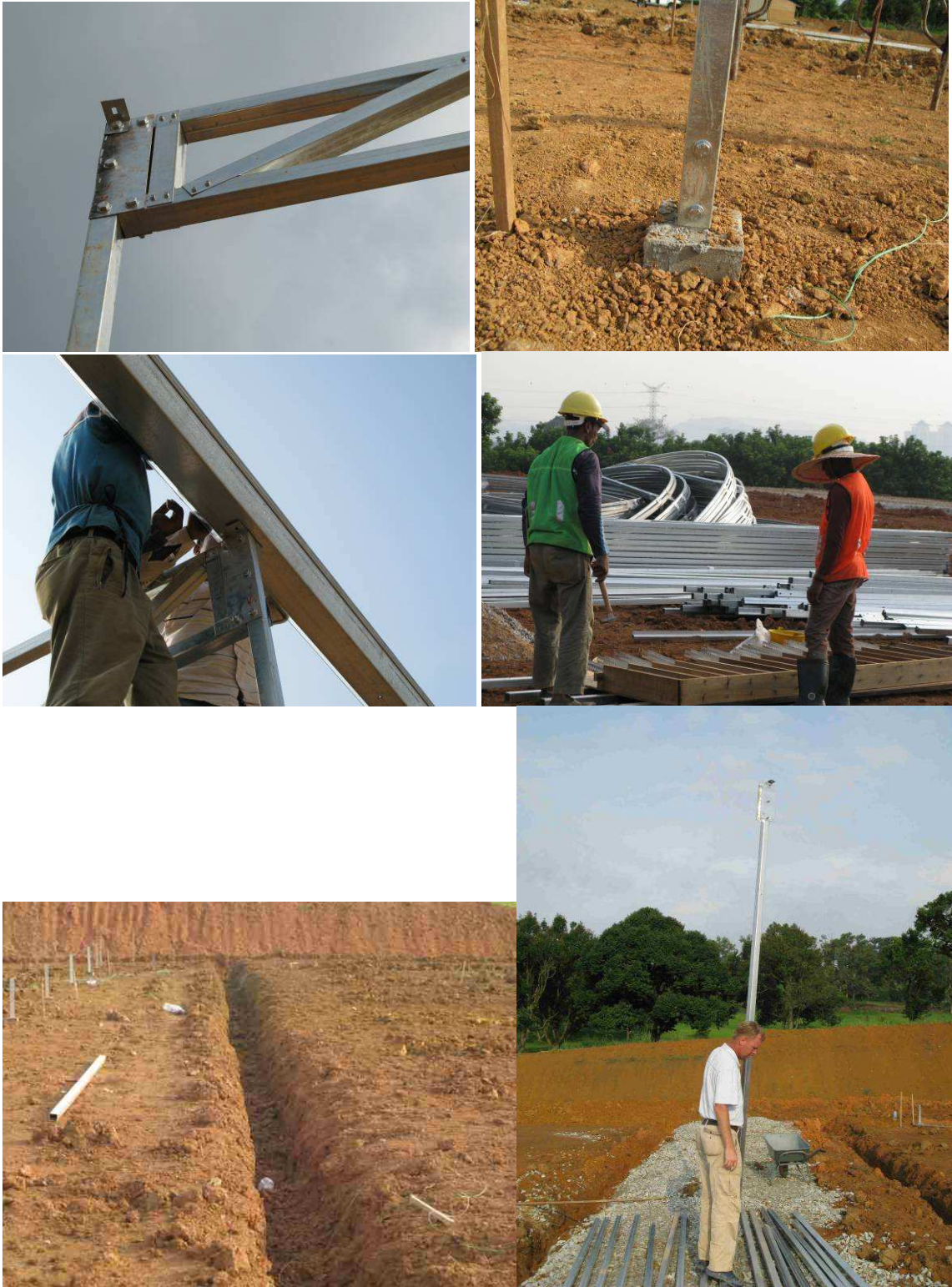
Figure 2. Some more images of the construction of the demonstration greenhouse at Serdang. Below right: Mr. Luuk Runia.
