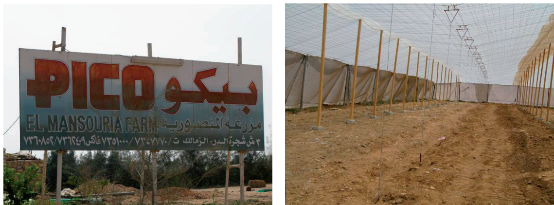
Figure 2. Road sign of Pico Farm (left) and interior of greenhouses under construction (right)
