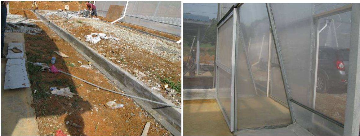
Figure 4. Trash around the greenhouse should be removed (left); the sluice in the greenhouse that must prevent insects from entering (right)
