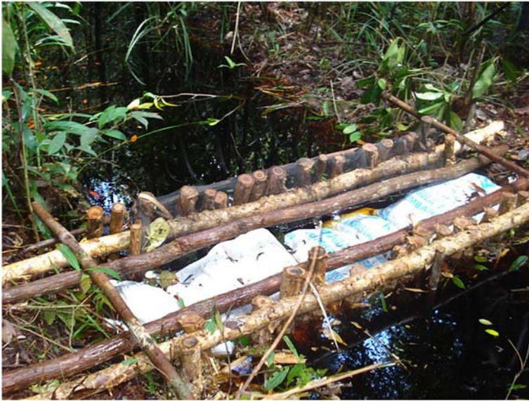
Fig. 9 Simple dam in the Bangah catchment made of locally available material (3 m long, 1 m wide and 2.5 m deep)
