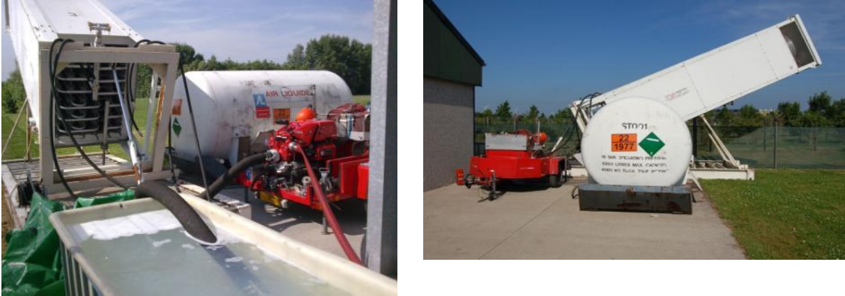
Figure 14 Liquid nitrogen tank, vaporiser, pump and pre-mix tank
