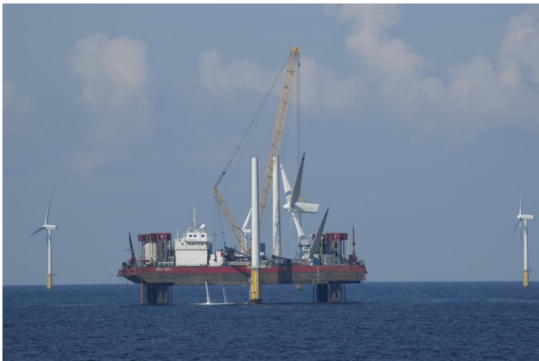
Figure 6. Construction activities in PAWP: preparations for hoisting a turbine. Building PAWP took place while OWEZ was already fully operational and while T-1 seabirds surveys (see main text) for OWEZ were conducted. Photos: Hans Verdaat, IMARES (top) Kees Camphuysen, NIOZ (bottom).
