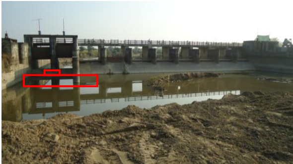
Figure 3: Hollow formed area at U/S floor
