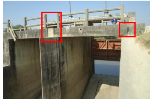
Figure 4: Increased gap in bridge deck slab joints
