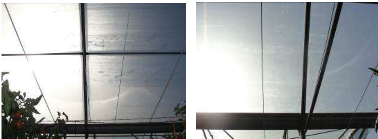
Figure 4.11. Left, control film showing condensation in the morning, and right, NIR_film, without condensation.
