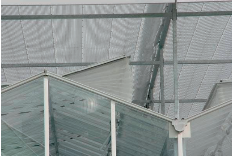
Figure 3.11. Insect nets in the window opening, combined with an external shading screen.
