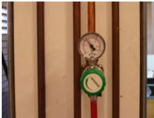
Figure 14: Fixed N 2 gas supply system at DLO-FBR was used for plasma trials.
