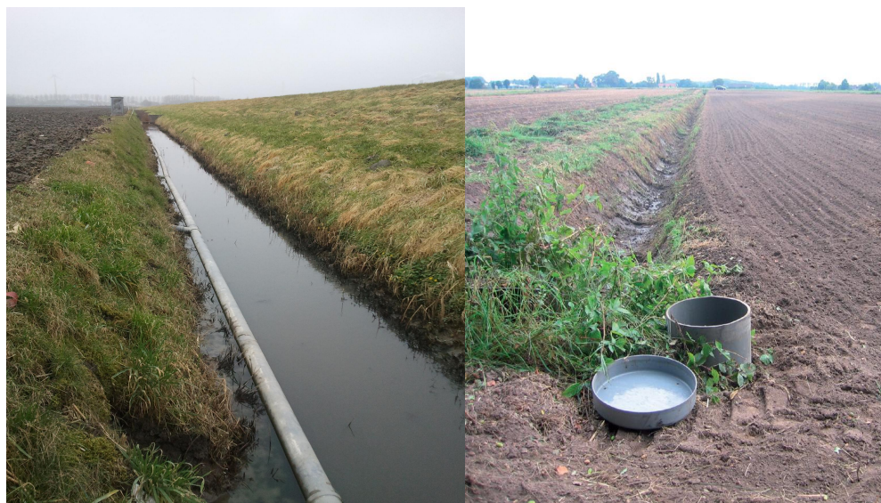
Figure a) Controlled drainage installed in fields in the Netherlands, where the drains are connected to a collector drain; b) and a vertical pipe which acts as the control unit for the water level.
