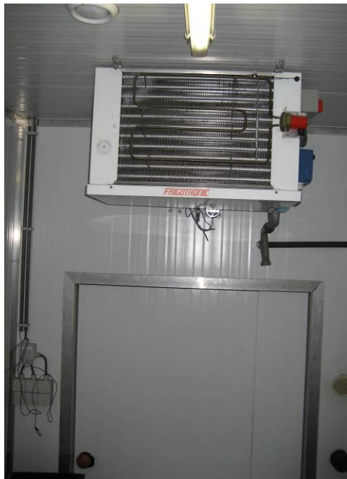
Fig. 11 Air cooler in climate room.
