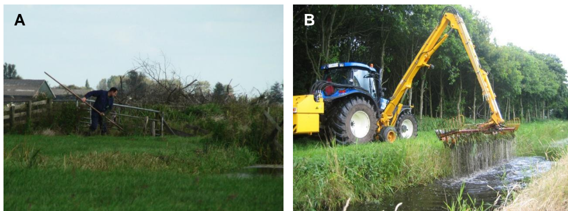
Figure 3. Ditch cleaning by hand with simple equipment (A) and modern ditch cleaning using powerful machinery with high removal efficiency. (Left photo: J.P. van Zuidam, right photo: H. Hoogenboom.)
