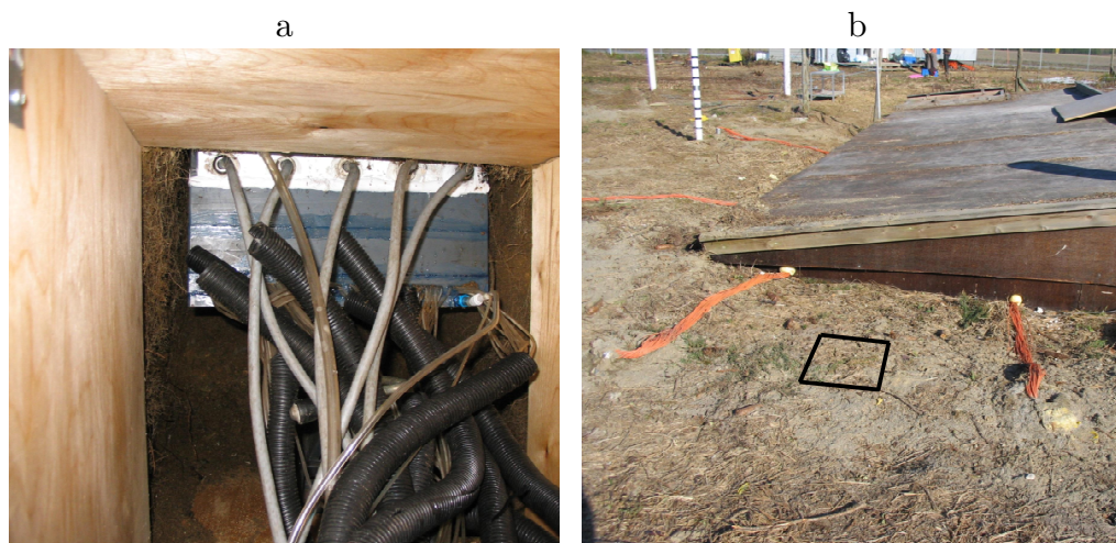
Fig. 1. Experimental setup. Installation of the multi-compartment sampler (MCS), shown from the trench (a). The location of the MCS shown from above (b). The marked square indicates the location of the MCS, 51 cm below soil surface. The roof of the trench is visible in the background. The width of the MCS is 31.5 cm.
