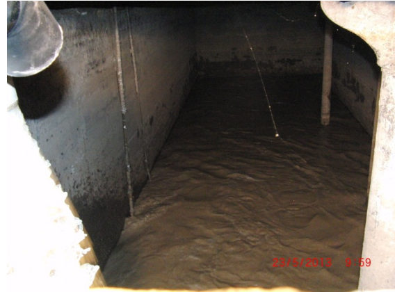
Figure 43: Storage vessel for the process water containing the fibres.
