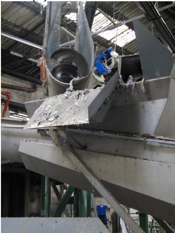
Figure 42: Screw feeders in the recycling plant.
