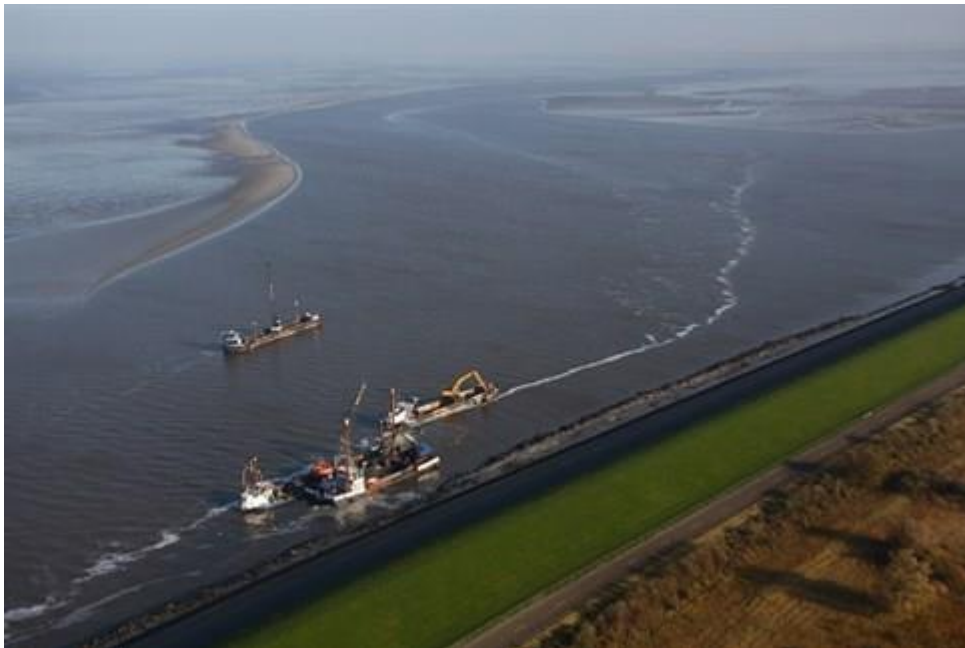
Figure 3.11: Morphologic dredging and protection of the dike near Vierhuizergat a channel which came perilously near to the dike (source: site Hoogwaterbeschermingsprogramma).
