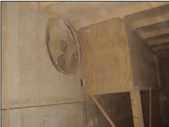
Ventilator 4 in de drukkamer
