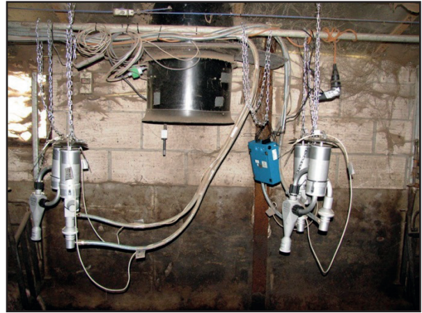
d. Measurement at the inlet of a ventilation shaft
