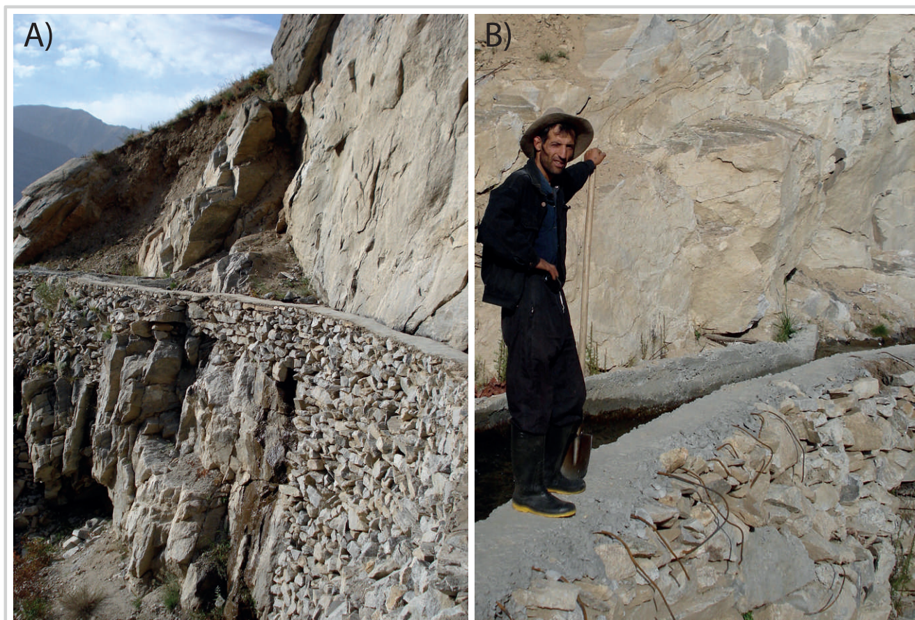
FIGURE 3 (A) Canals are often situated on steep slopes; (B) they require a great deal of maintenance. (Photos by Lisa Bossenbroek)
