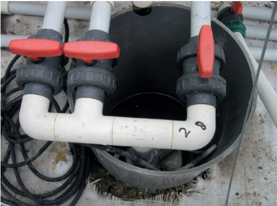
Photo 1 The drainage tank half under the ground in the greenhouse collects the drainage from two plant rows. The water from the drainage tank was pumped to an irrigation tank in the technical corridor outside the greenhouse. This was controlled by a float valve in the drainage tank.
