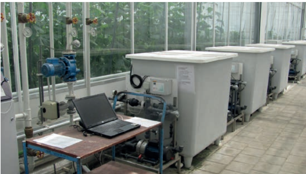
Photo 2 Irrigation tanks in the technical corridor outside the greenhouse. Irrigation was controlled by computer and was scheduled to reach on average 25% drainage water on a daily basis.
