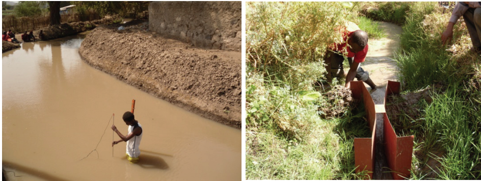
a. Current- metering for Q - h relation in a diversion canal at Golgota Scheme b. Parshall flume installation at command head at Wedecha Scheme Figure 8.8. Measurement of water delivery in irrigation canals
