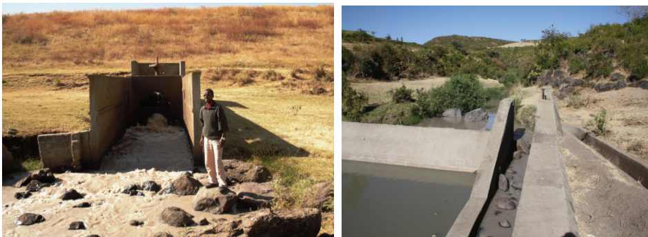
a. Wedecha Reservoir outlet b. Diversion structure to Godino sub-system Figure 3.6. Water acquisition and control structures for Wedecha Scheme
