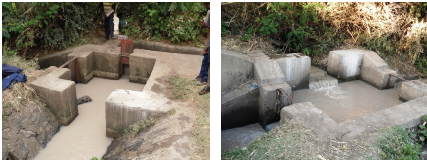
Figure 9.5. Water division structures with demolished gates at Wedecha Scheme
