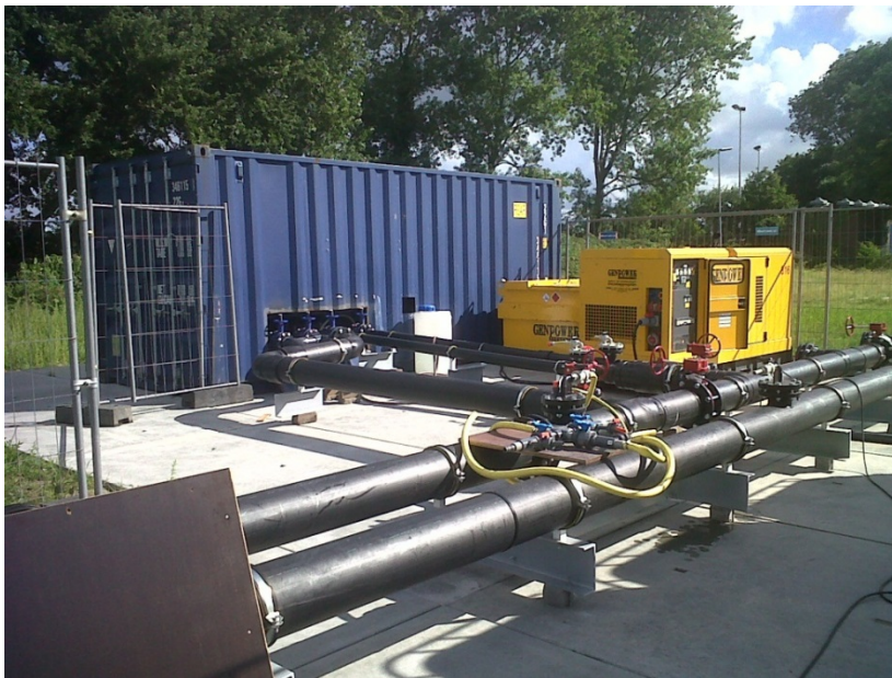
Figure 3 The BIO-SEA BWMS container connected to the main piping system
