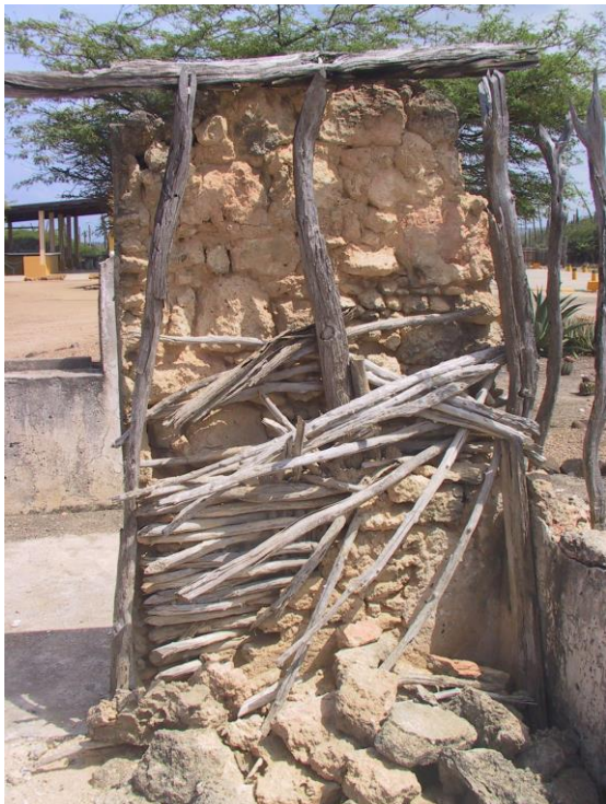
Fig 2.2: Example of a structure of cultural and historic significance inappropriate for restoration. The goal in this case is stabilization and only under expert guidance (photo: A. Debrot).
