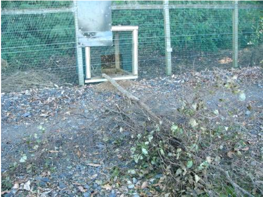
Figure 6. A ‘tree-fall’ hole, with cover removed. This breach type was open for 24 hours at a time.
